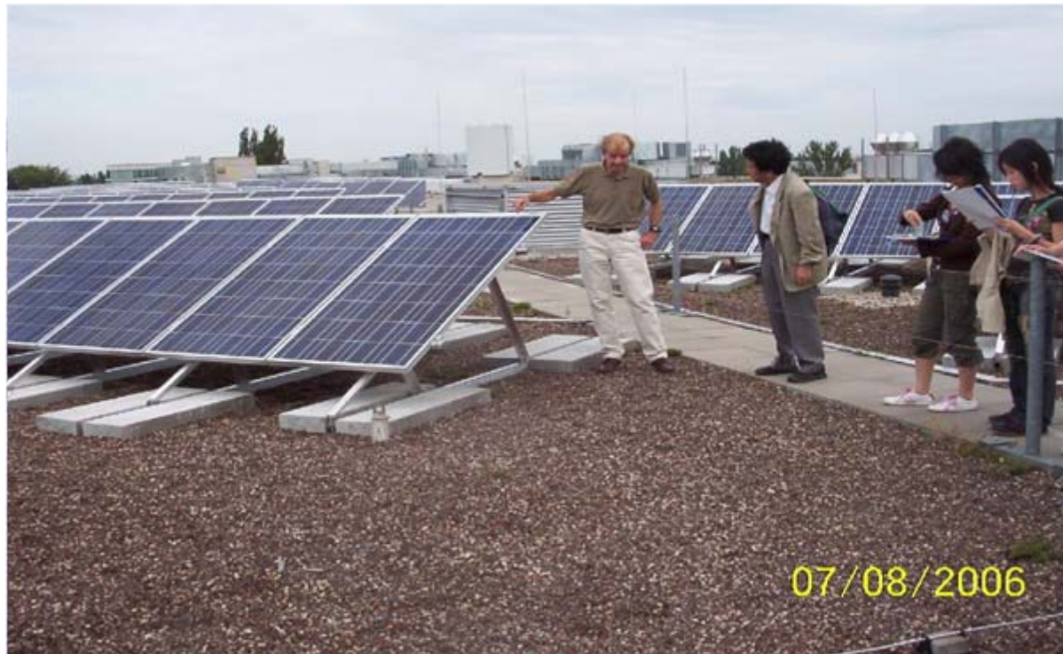
Roof of the Environmental Center, 48 kWp, poly-Si modules by SOLON. installed in 2006, owner: DACHLAND GmbH
